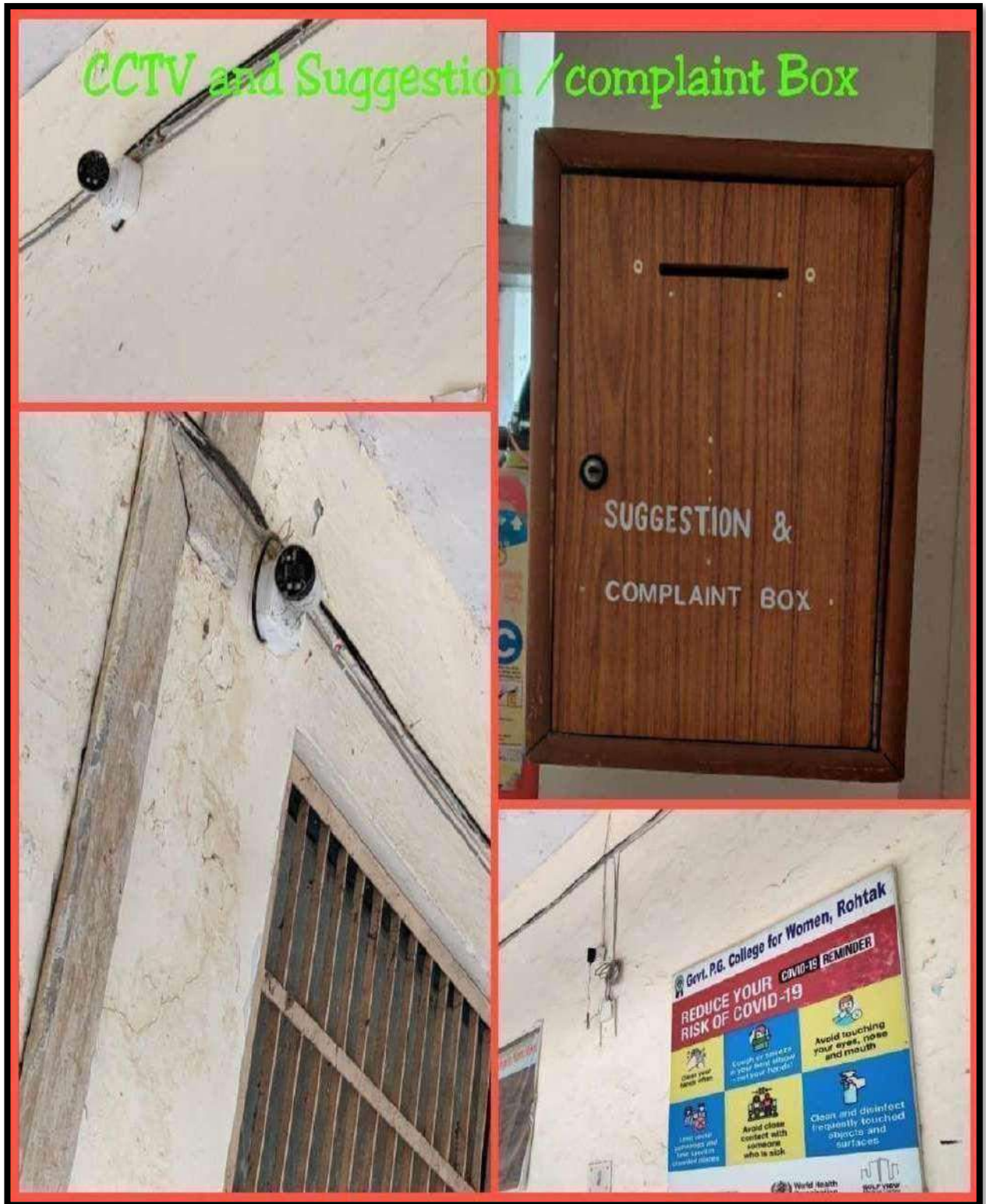
CCTV and Suggestion/Complaint Box
